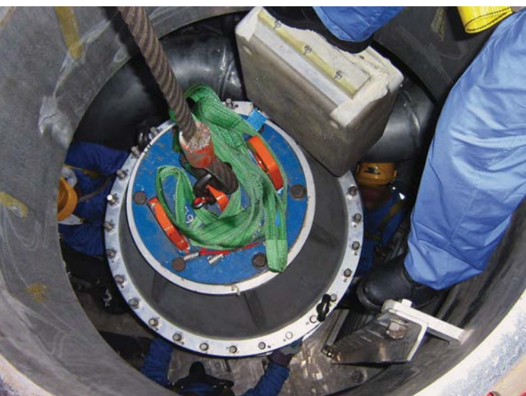
Lifting an Ebara cargo pump clear of an LNG carrier tank for servicing
