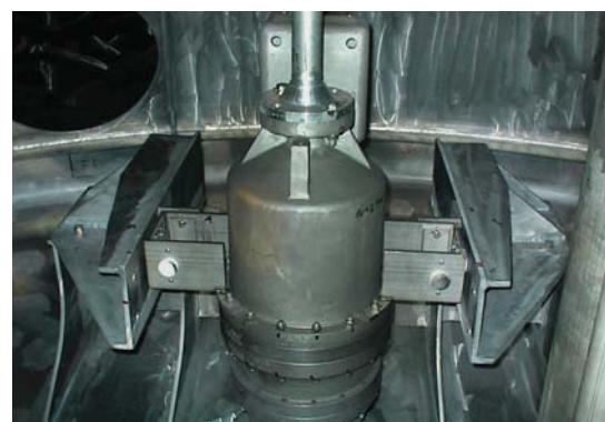
In addition to two cargo pumps each LNG carrier tank is provided with a spray pump
